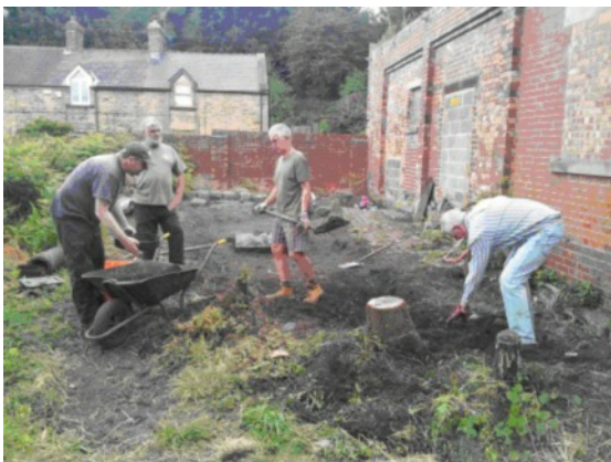
Photo:- Stumped! Digging up to/around tree stumps Cue: the practical engineers. The group is fortunate to count a number of very handy folk amongst its number: engineers, surveyors, geologists, mechanically-minded and ready to provide solutions when
