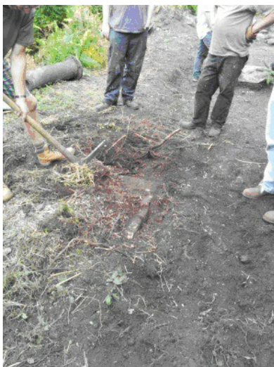
Photo:- Corner of the wall - dressed outer stone with thin rubble inner.
