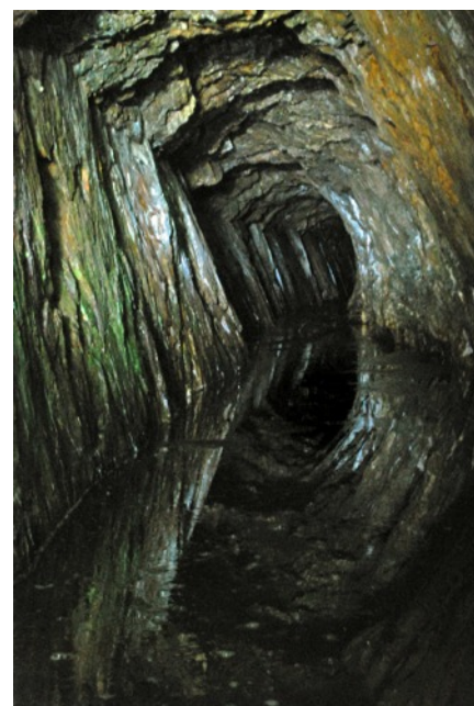
Photo: By directing the beam and painting the light
