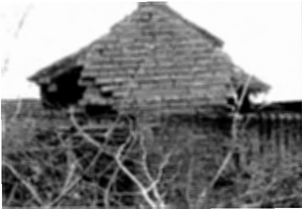
Photograph 2 The falling of nearby trees unsettled the office gable, on the nearside to the A65.
