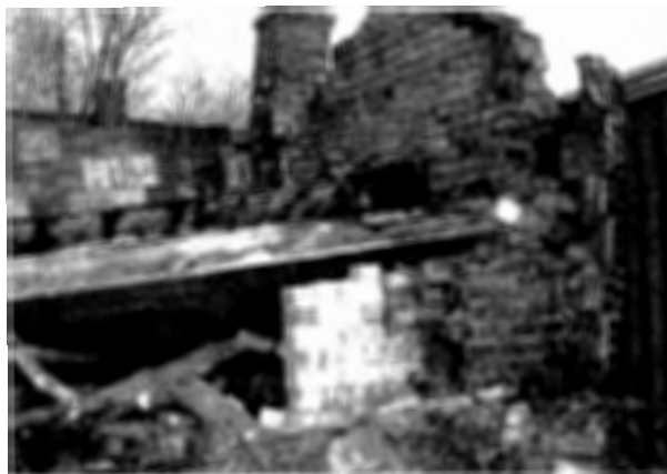
Photograph 3 Alterations within the yard caused the next and final stage of collapse.
